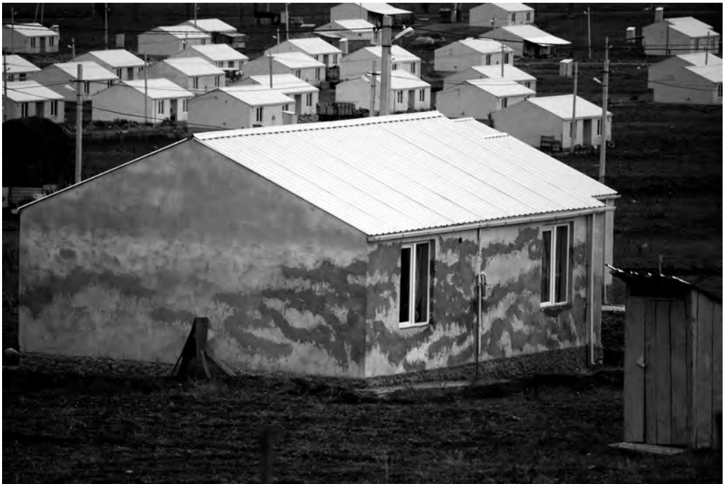
Prezeti settlement, where the chaos of aid appeared in material form, as the newly built cottages began disintegrating almost immediately.
